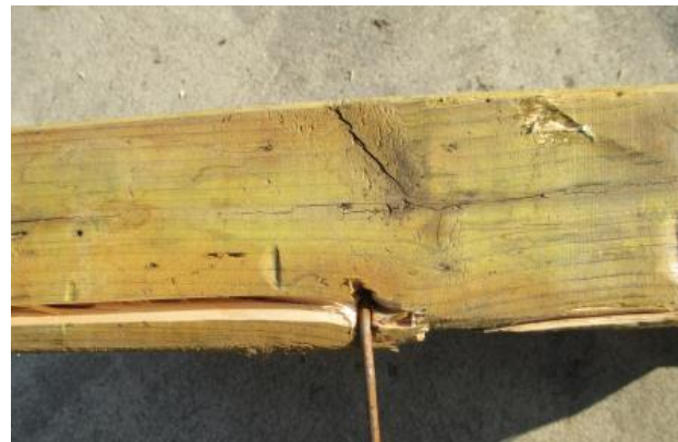
Damages caused by nails
