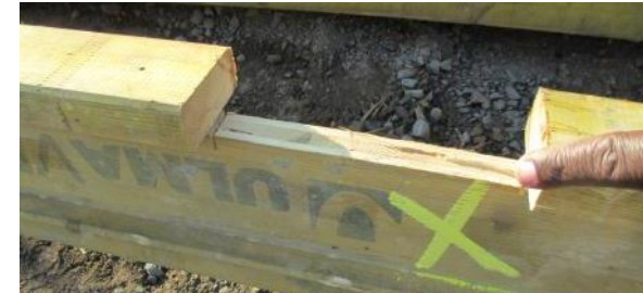
No cutting in girder
